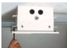
Adjust to ensure ceiling integrity
